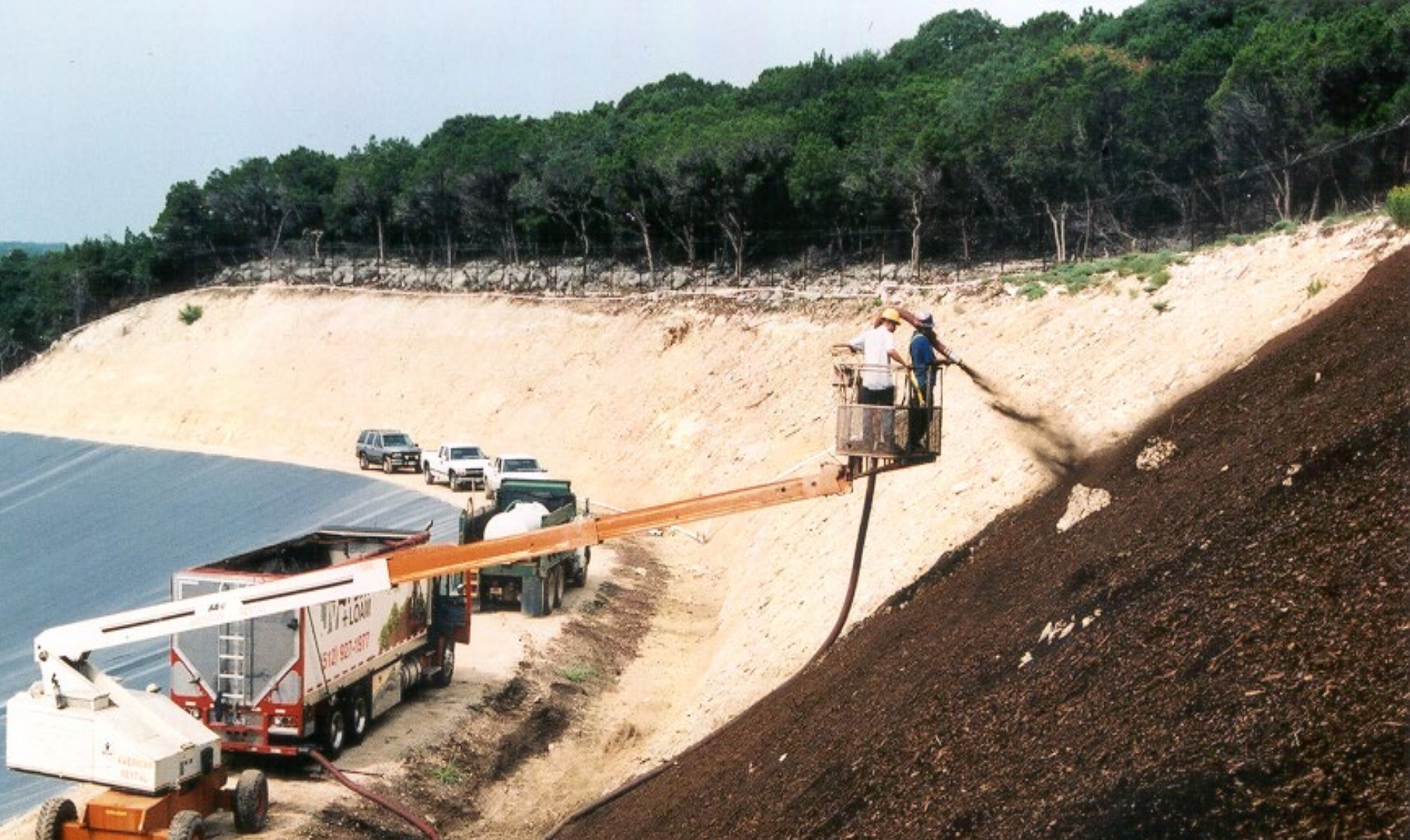
Application to 1:1 ROCK SLOPE 2" compost mulch w/native seed mix Barton Creek Development – Austin, TX AUGUST 17, 2002
